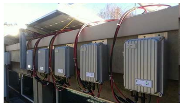
Figure 2: View of the DC/DC converters for individual PV-modules on the roof of HES-SO Valais-Wallis
