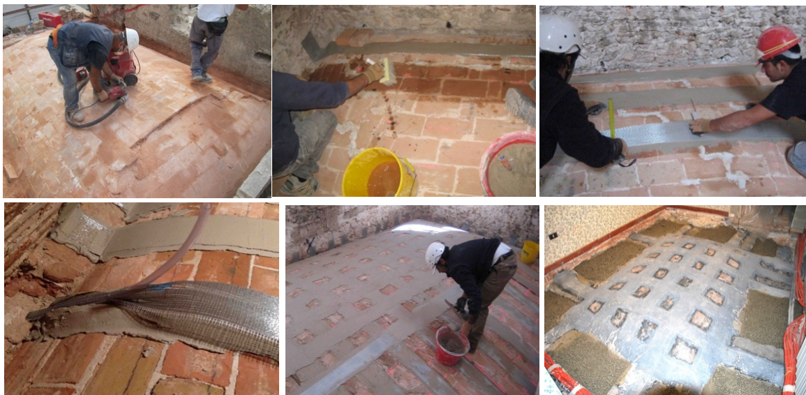
Figure 1. Phases of strengthening brick masonry vaults at the extrados: a) preparation of the extrados of the vault after the removal of the filling; b) application of a primer for enhancing the bond between the extrados of the vault and the inorganic matrix; c) application of the Ultra High Tensile Stress Steel strips; d) end connections at the abutments; e) application of the covering layer of mortar matrix and of a second transversal set of strips; g) construction of brickwork spandrel walls for the backing and filling with granular material.
