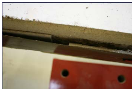
Figure 3. Debonding of EBR CFRP laminate after fatigue loading (REX20-H)
