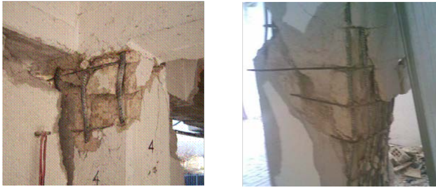
Figure 1: Damaged columns from L'Aquila earthquake (Del Zoppo et al. 2016,a)
