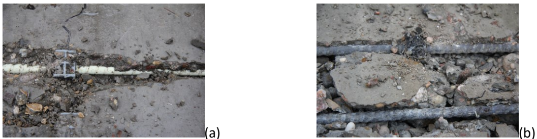
Figure 11. Post-heating bending. Rebars after failure of the panels with 5 cm concrete cover: (a) Schöck ComBAR and (b) FiReP Rebar P.
