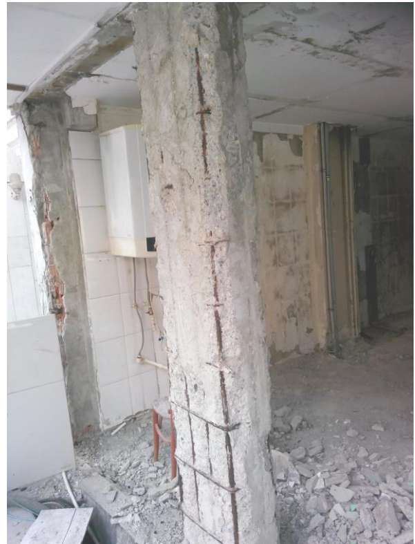
Fig.2 - Corrosion Damage on Columns
