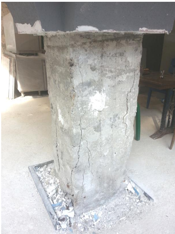
Fig.3 – Cracks on Corner Column
