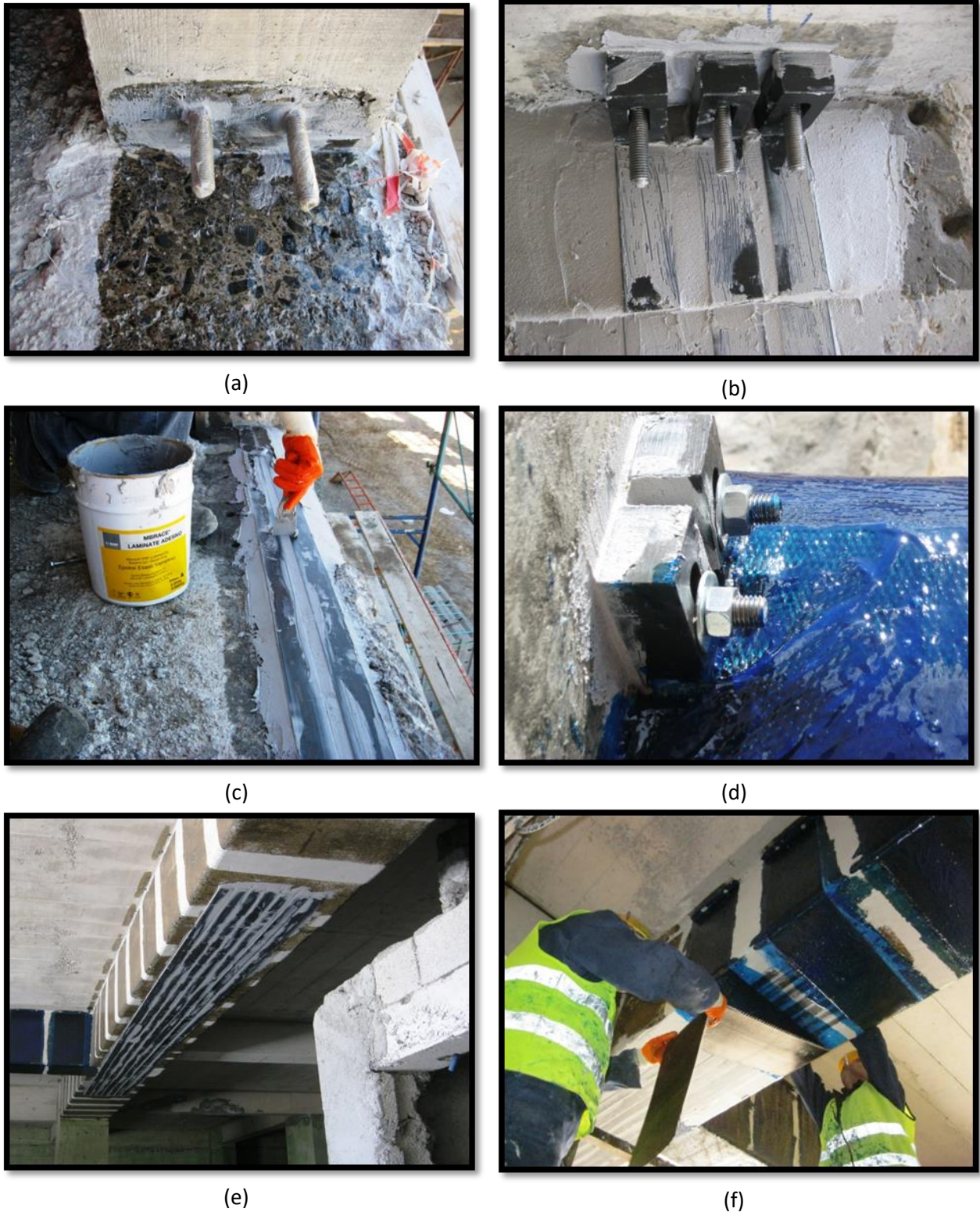
Figure 4: Flexural strengthening of beams a, b, c, d negative moment strengthening application, e, f positive moment strengthening application (f is also represents the shear strengthening application)
