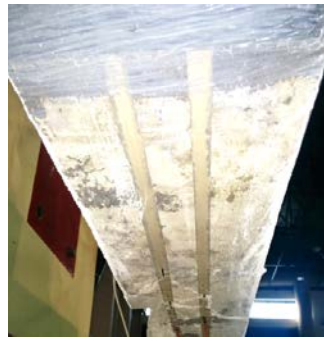
Figure 4. No debonding occurred in the case of NSM strengthened beams after fatigue loading (RNSM40-H)
