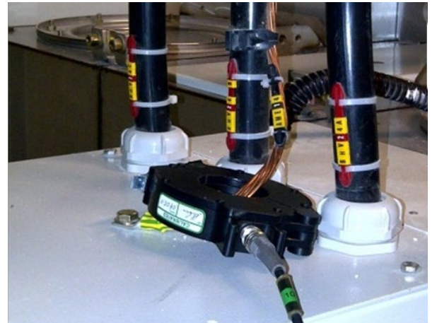
Fig. 6. Measurement of PD signal with HFCT at HVPD Ltd.
