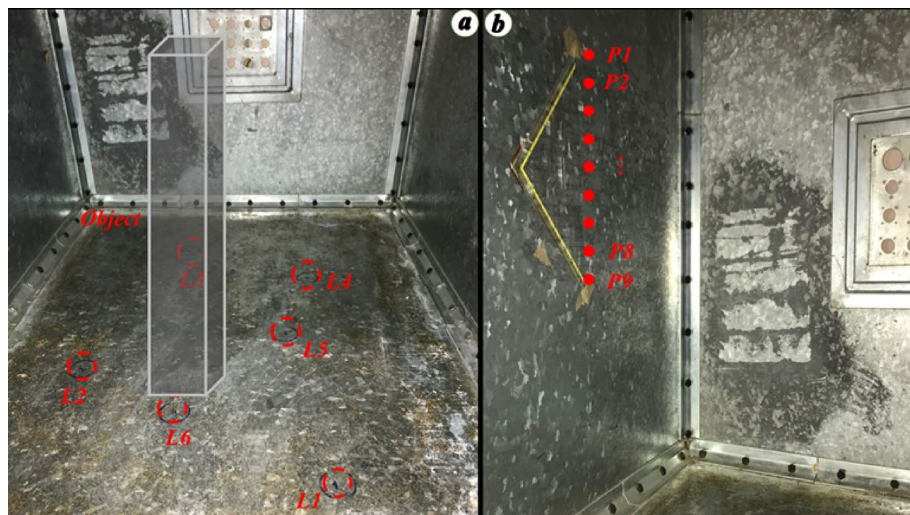
Figure 8. Assumed PD locations. (a) On the floor of the tank ( L_1, \dots, L_6 ). For better illustration, the metallic object was removed temporarily and replaced with a translucent parallelepiped, (b) On the left-wall of the transformer tank, P_1, \dots, P_9 are spaced 2.5 cm from each other.
