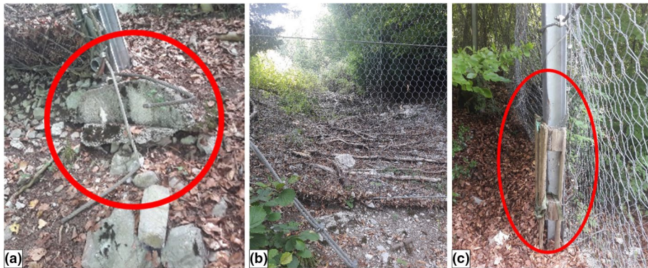
Fig. 11 Inspection of barrier fence G4. a Signs of erosion at the foundations due to rainwater; b different types of materials located in close proximity of the fence; c trace of impact of a boulder on one of the posts
