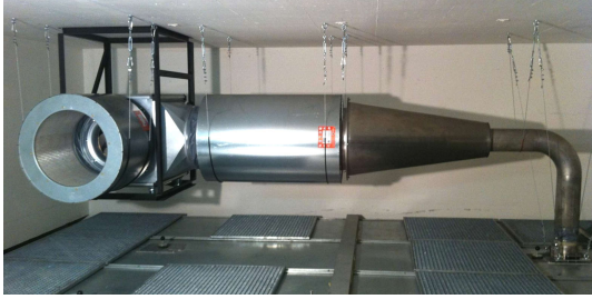
Figure 4: Wind tunnel setup in the machinery room above the anechoic chamber.
