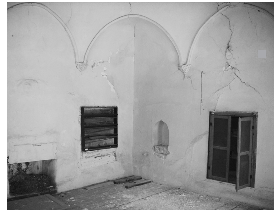
Fig. 3 North-West corner before restoration, fire place, two windows turned into a cupboard and a niche.
