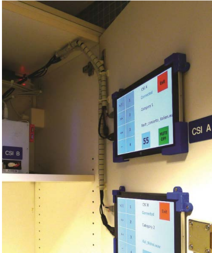
1b. Control system
