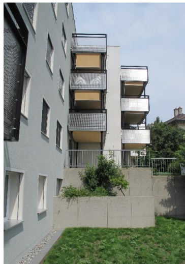
Figure 7 Trois-Portes 61-63: Insulation of the envelope, enlargement of the balconies and installation of 60 m 2 of thermal solar panels (Archetype 4, Renovation type II). Pictures from architect.
