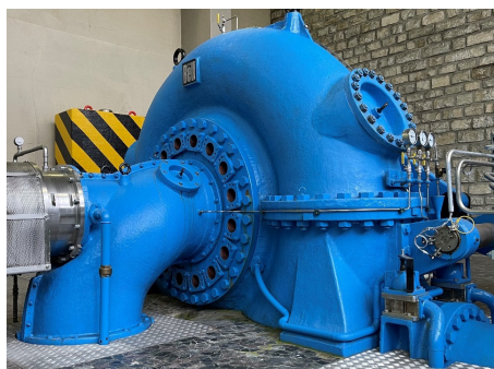
Figure 2: The double-runner Francis turbine at Ernen hydropower plant in Wallis, Switzerland.
