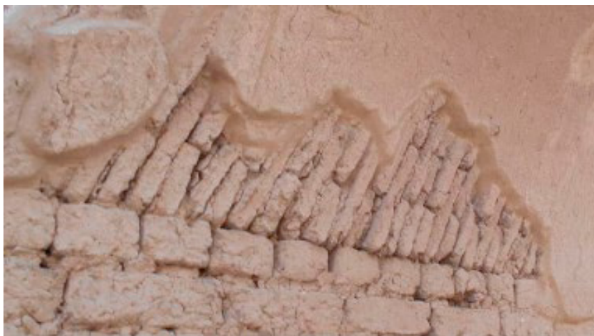
Fig. 1. Mud-bricks laid tilted in an Ancient Egyptian barrel vault (in the storerooms of the Ramesseum temple). from (El-Derby & Elyamani, 2016)
