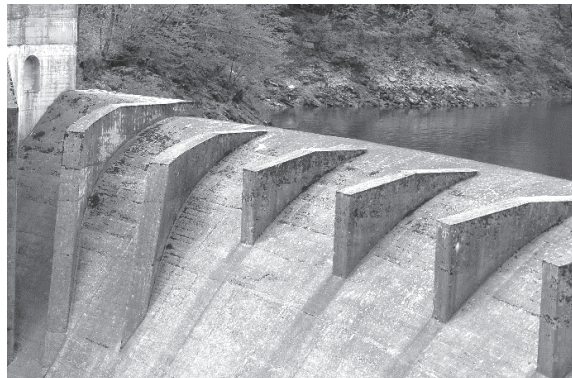
Figure 11. Photo spillway inlet (standard weir) of the Palagnedra Dam in Switzerland with the removed piers.
