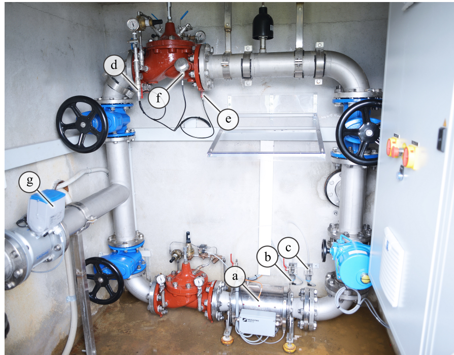
Figure 11. Installed DuoTurbo pilot in a drinking water supply network at Savièse (VS Switzerland). The positions (a–g) refer to the instrumentation list given in Table 7.
