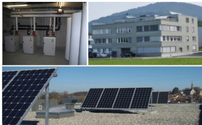
Fig. 2. Pilot site - RUIDA building in Switzerland
